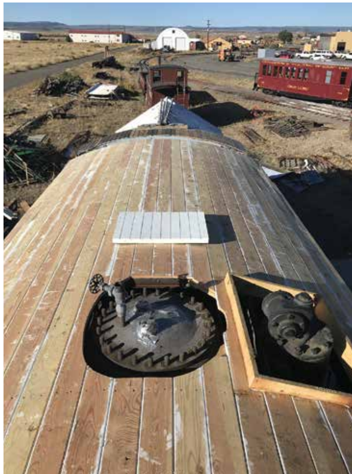
View from the roof: The complexity of framing and building around the steam dome and air pump is evident.
