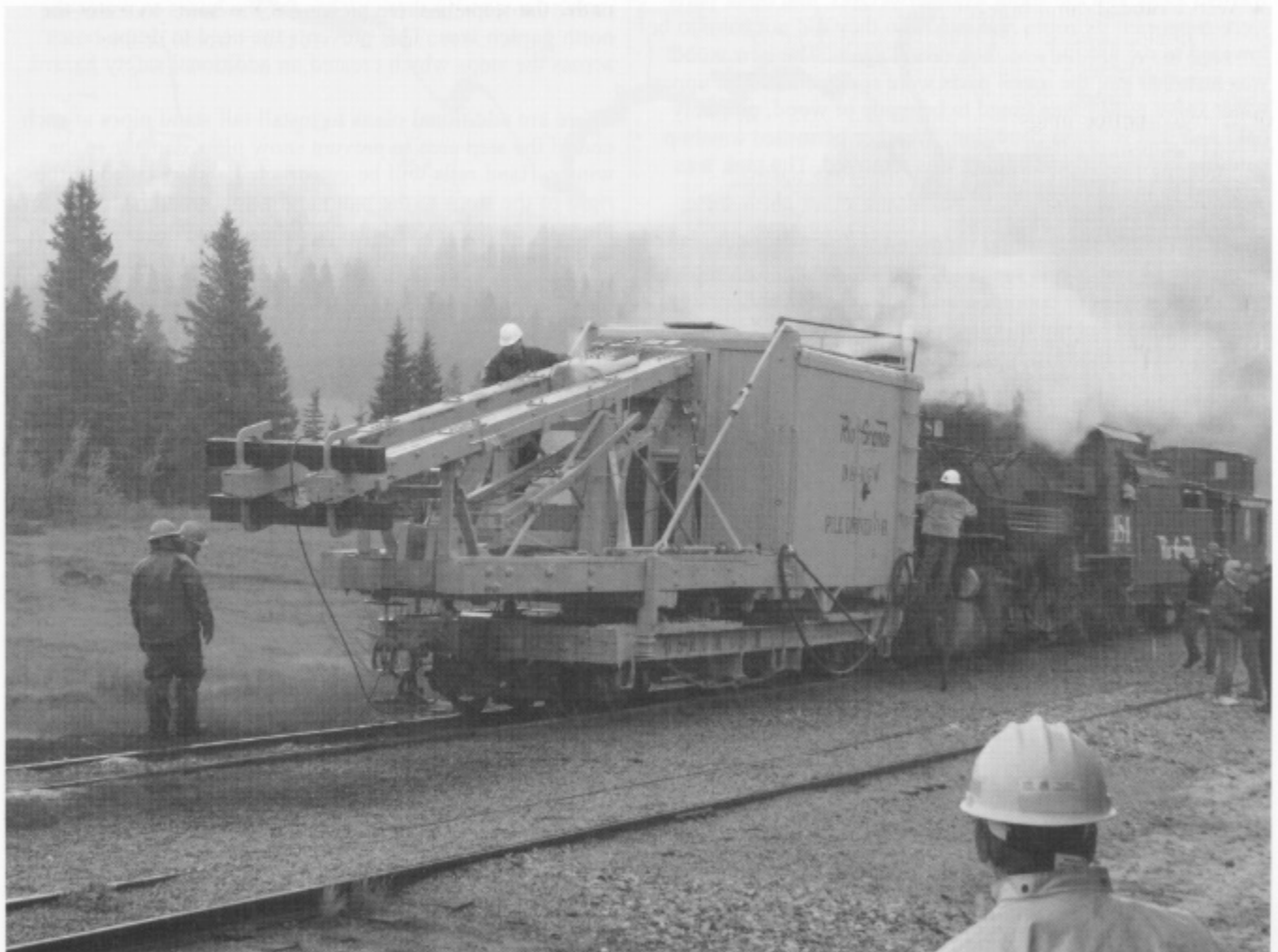
In a scene that was probably common early in the last century, the crew of pile driver OB works in heavy rain to set up the pile driver at Cumbres on June 20, 2009. (David Lee)
