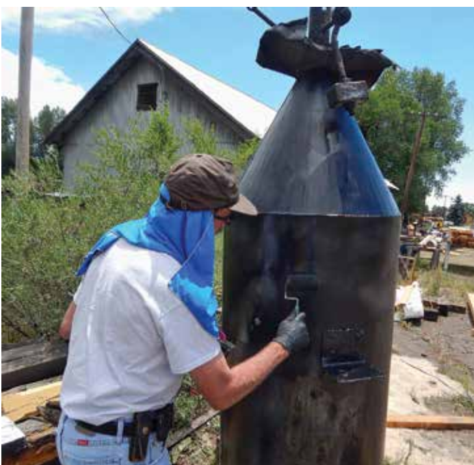
The compressed air tank (top), the cyclone tank (bottom, tank inverted) and the air/sand mixing tank all received scraping, sanding and paint before they were reinstalled in the Sand House.
