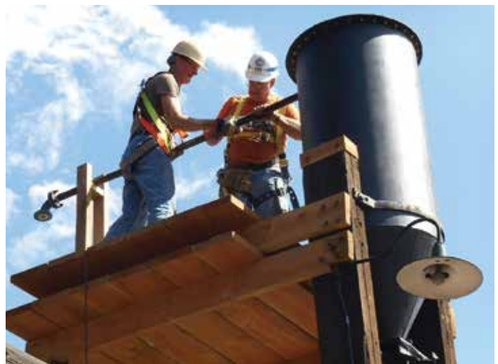
(Top) Up she goes! (See Dispatch cover) Once the crane had lifted and placed the cyclone tank in its nest on the tower, the air/sand mix line was attached from the tank below.
