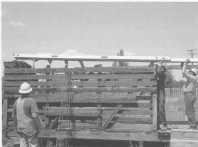
Kevin Corwin, Warren Ringer, and Dave Traub place finished top sill on left wall, B end of car. Dan Pyzel is watching.
