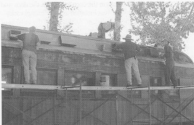
Painting the repaired roof of Milwaukee business car 222. From left to right: Valley Lowrance, Tarry Rahne, John Cole, and Warren Ringer.
