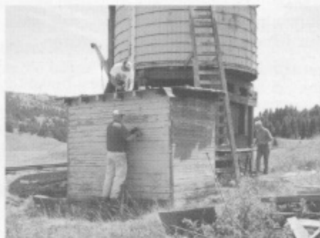
Yancey Juergenson is securing new pine roof sheeting. Tom Gregory is scraping paint. Don Juergenson is cutting sheeting to size.
