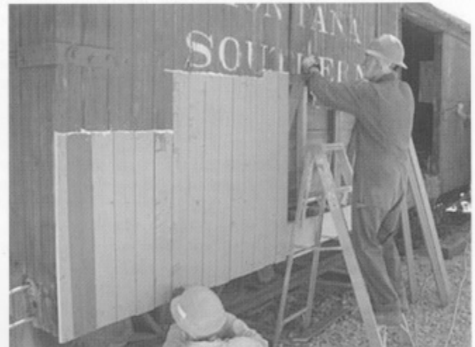
Warren Ringer and Irv Milheim replacing siding where it had to be removed for installation of a new side sill.
