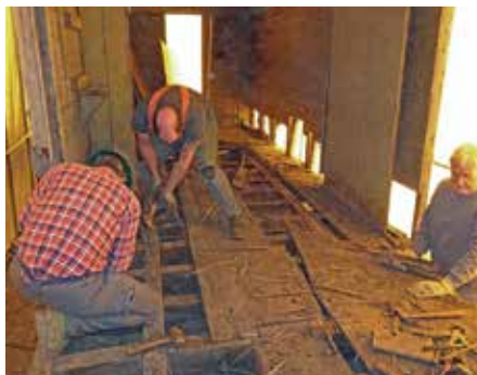
The interior floor was removed which exposed both the frame and original 1881 wood-shaving insulation.
