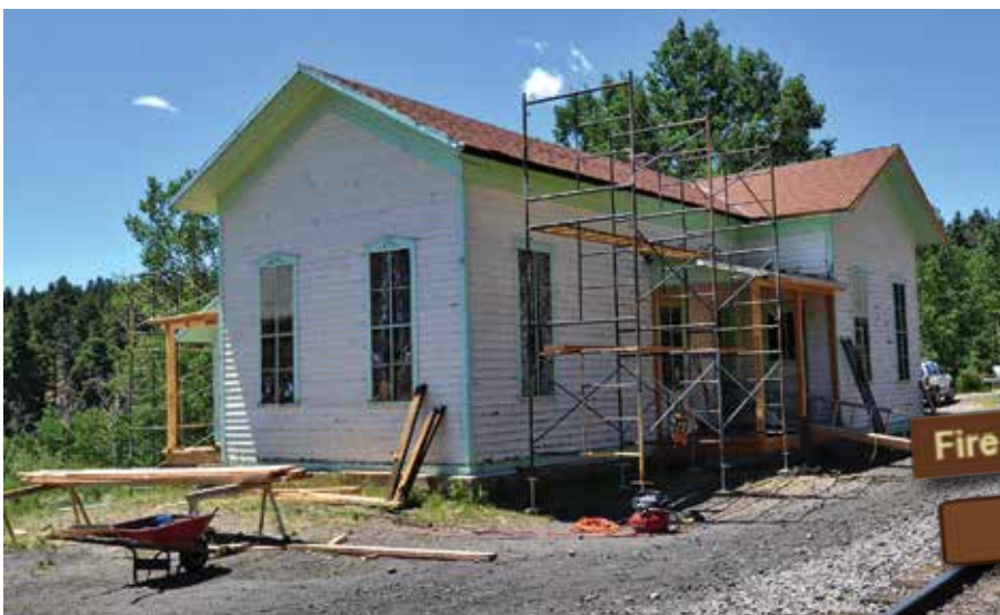
The roof of the Sublette Section House was in serious need of repair and restoration, but access to the site was through national forest lands, was closed to any access.
