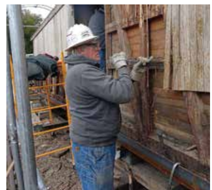
Removal of the rotting siding revealed needed structural work.
