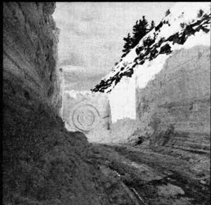
ONLY when the wing started scraping the rocks at the right did the crew realize that the rotary had derailed here. Rerailing was not a problem: the rotary was backed out and the wheels always followed the flange marks in the ice and came back to the rails.
