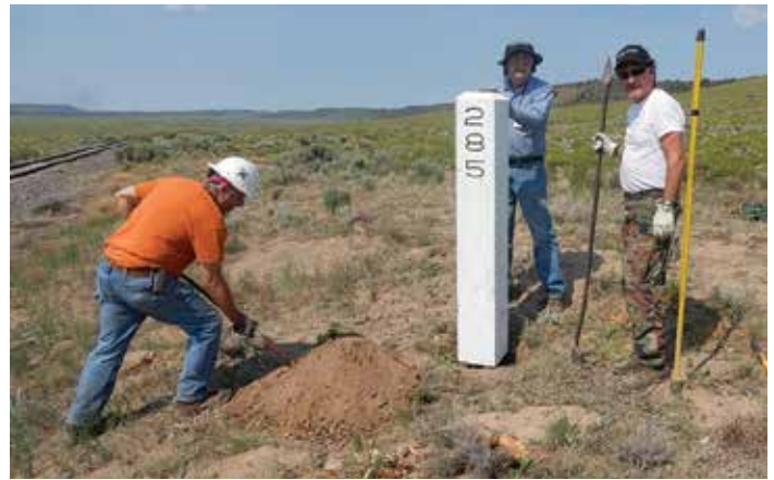
(L to R) Sign crew members Paul Davenport, Terry Woolsey and Mike Mahoney replant Milepost 285, five miles southwest of Antonito, after some needed maintenance. Photo by Jim Gross
