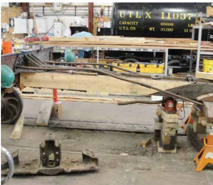
Two wood beams have been cut away from the steel channel on BOTH sides because of wood rot, and one new piece has already been inserted. To gain access, the last cross frame had to be removed, the truck had to be rolled away and the truck bolster had to be removed. The bolster is the large casting in the lower left corner of the photo.
