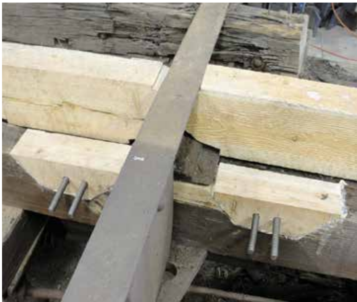
Two wood inserts have been glued into the outer frame beam. Expanding glue is used to preclude having gaps where water can collect and cause more rot.
