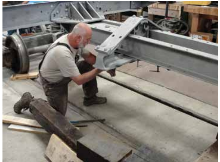
This photo shows the steel end sill and the steel frame channels with the wood beams removed. Ron Senek is preparing to remove the truck bolster so that new wood frame beams can be installed.
