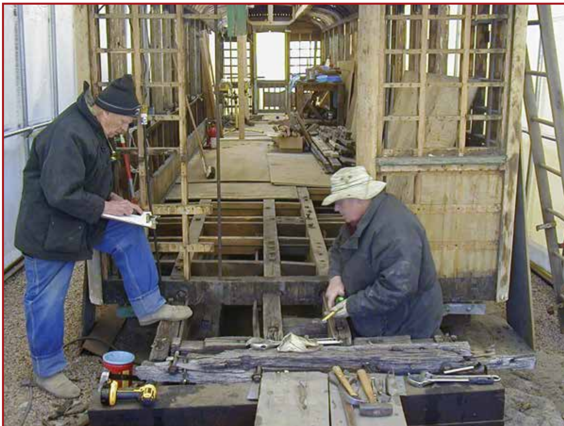
Glenn Hall and John Eng measure and take notes on the construction of one of the end platforms of Pullman Tourist Sleeper 470 near the beginning of its eleven-year restoration. Photo by Duncan Burdick
