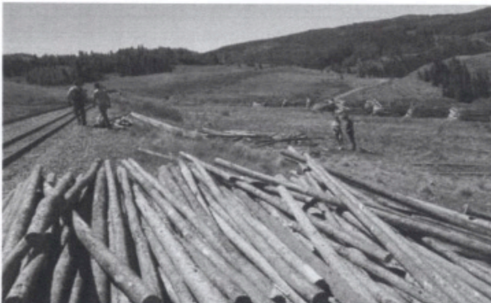
Emmanuel Lopez, Gabe Karns, Bernadette Karns and Maggie Karns prepare to haul logs from track side to the fence site.
