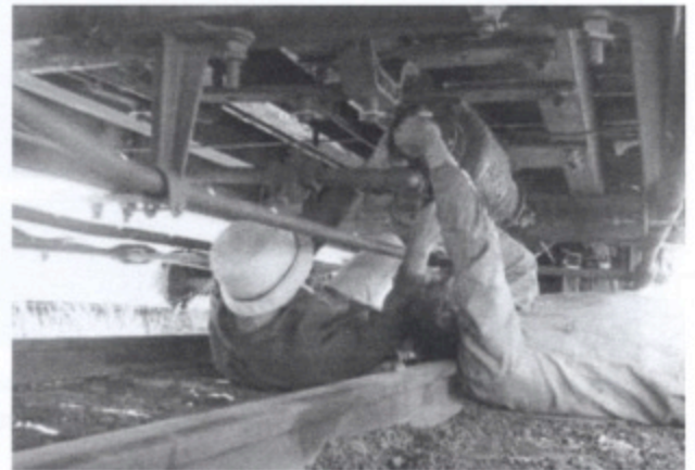
Clyde Putman and TL Art Randall installing a triple valve on Car 1648.
