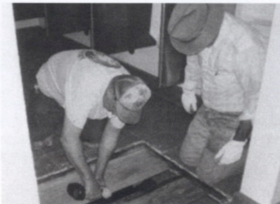
Tim Bristow observes Bob Reib attaching a nailer to a floor joist.
