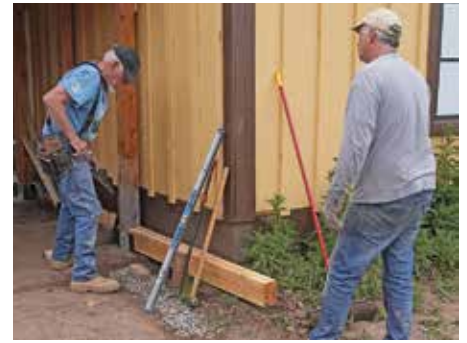
Proj. 1408: SHPO - General Repairs to Exterior of Osier Depot including windows, trim, and siding. Sessions C & D
