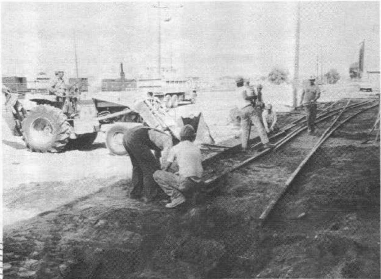
One of the most significant projects tackled by the Volunteers was the removal of the last 400 feet of dual gauge track in Alamosa, Colorado, including a dual gauge switch. Here Volunteers carefully remove the switch for future reinstallation in a dual gauge display in Antonito. L to R: Julian (on tractor), Wade Hall, Leo Schmitz, Cal Smith, Jim Herron, Jason Rupley, David Hoyt and Clay Wilson. August 17, 1989. Photo by Peter Smith. (See story by Cal Smith starting on page 8).
