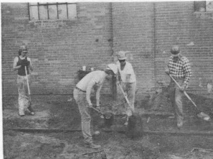
Left: Volunteers uncover buried 3-Rail Track along side PSC power plant (L-R: Jason Rupley, Clay Wilson, Cal Smith and Jim Herron) Alamosa, August 17, 1989.
