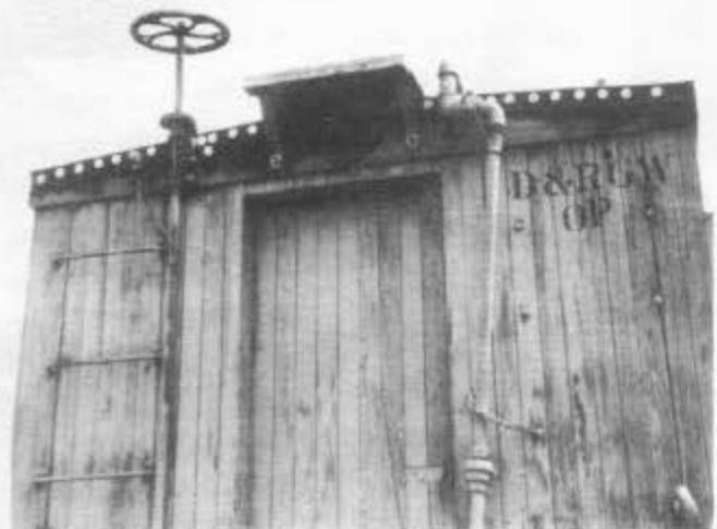
ABOVE: End view of derrick OP showing new braces for roof walk, steam pipe, and reinstalled brake wheel and staff with ratchet and pawl. The edges of the new roof are tacked to the fascia board with nails and roofing washers. The roofing crew for the derrick was Howard Bunte, team leader; Dennis Chiles; Jack Schuh; and Craig Story. The crew also began work on historic caboose No. 0503, built in 1886. Old roofing material on the cupola was removed, a few boards were replaced, and new canvas and tar compound (Indukril) were applied. Photograph by Arthur Nichols.
