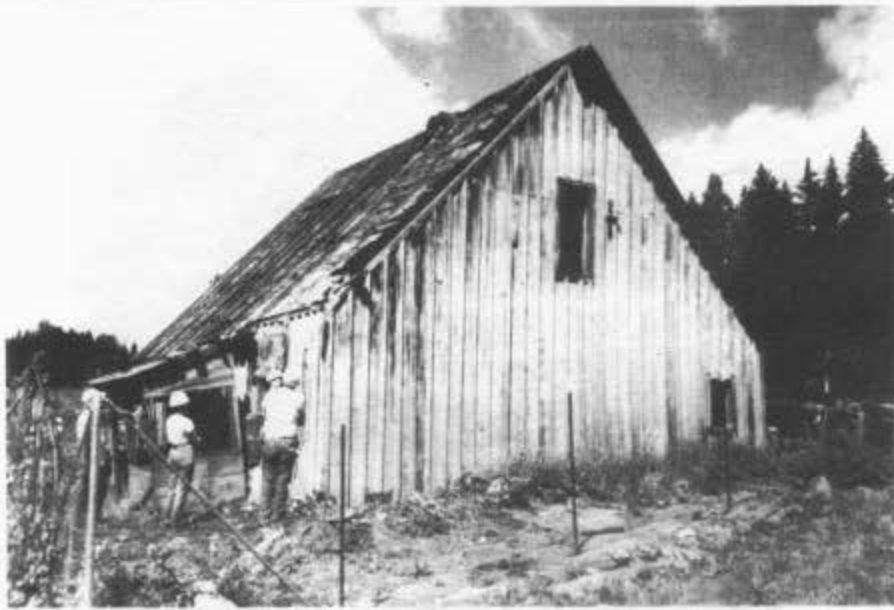
LEFT: Crew members inspecting the north side of the car inspector's house at Cumbres Pass. The stabilization of the house was started by installing two walls that were removed several years ago. John Rupley was the team leader at Cumbres. Crew members were Samuel Bjorkman, Thomas Bjorkman, Kyle Norcross, Ted Norcross, Jack Ryan, Casey Rupley, and Janet Rupley. Photograph by Arthur Nichols.
