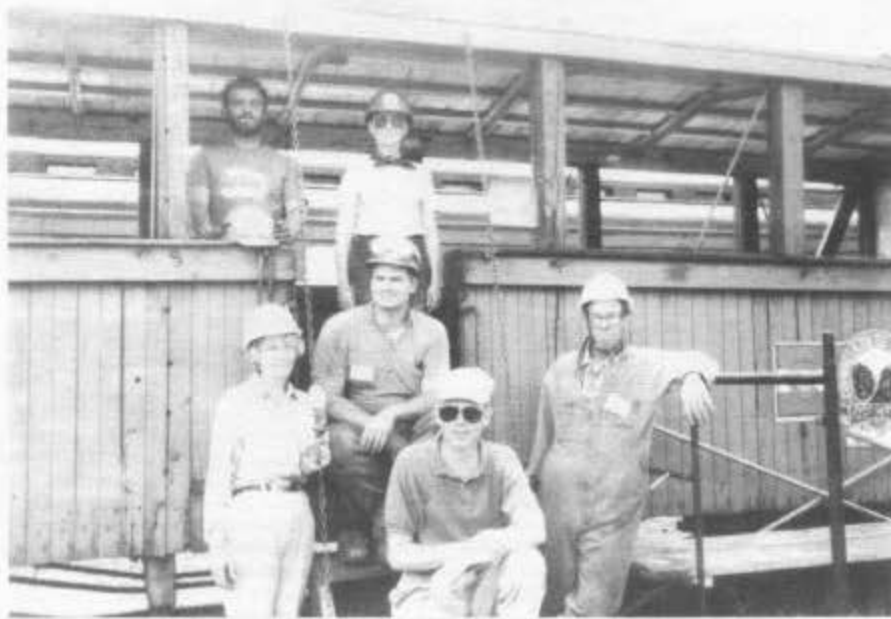
LEFT: Car repair crew. Passenger coach No. 203 was readied for service as the Moonlight Train snack car by removing the seats in the car, stripping the old and damaged flooring, and installing and painting a new plywood floor. New baseboard molding was installed, and several panels of sheathing below the windows were strengthened. Also, new Plexiglass windows were installed where needed. Standing in the snack car are Bill Kepner, team leader, and Theresa Shaw. Front row left to right are Martha Mackey, Ray Parks, Ben Fly, and Al Kilminster. Not shown are Marty Katcher; Shirley Russom; and the snack car crew for the Moonlight Train ride -- Tracy Griffin, Lori Hall, and Jill Saberhagen. Photograph by Arthur Nichols.
