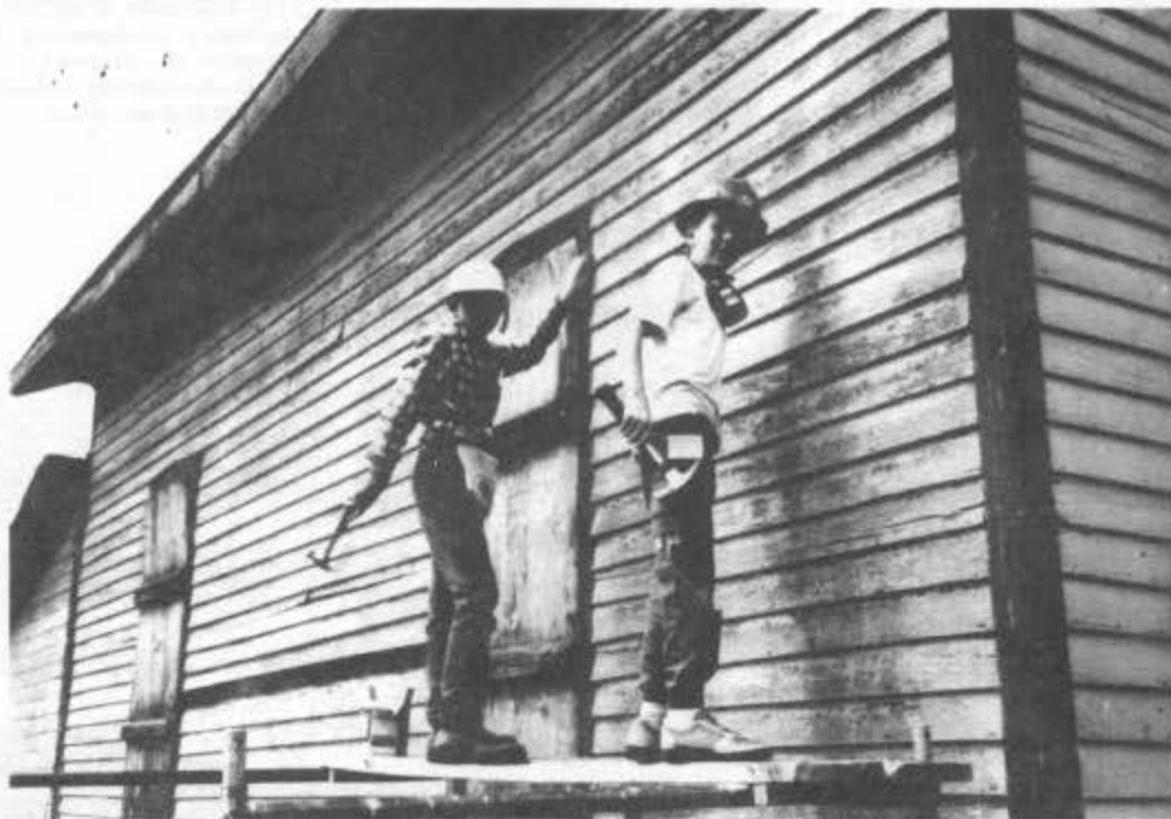
ABOVE: Young people play an important part in the restoration of the railroad. Here, Kyle Norcross, left, and Casey Rupley renailling siding on the section house at Cumbres Pass. Photograph by William Lock.
