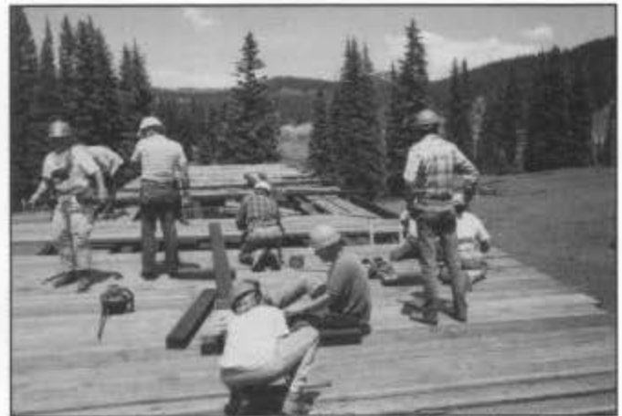
Cumbres: installing new 2 x 12 boards on the snowshed roof over bays nos. 4 and 5.
