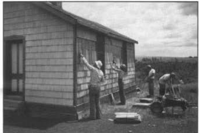
Sublette: installing new shingles on the west wall of the shingle bunk house; installation was completed at the work session.
