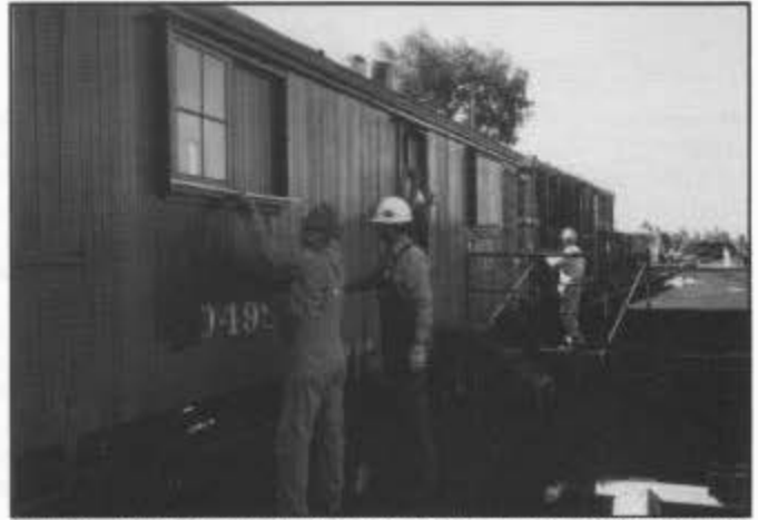
Chama: installing new screening on bunk car no. 04982; work was finished on two of the three bunk cars.
