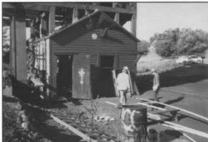
Chama: the coal tippie crew working on the north and east sides of the machinery room; new cedar siding was installed on the east side.
