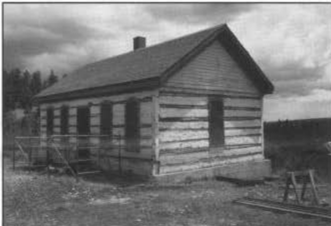
Sublette: exterior work on the log bunk house has been finished; new chinking is now in place.
