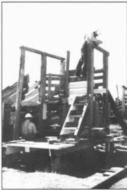
Repairs were made to the landings, ladders, and loading chutes of the stock pens at the south end of the Chama yard. August 1993. Photograph by Jessica Ratliff.
