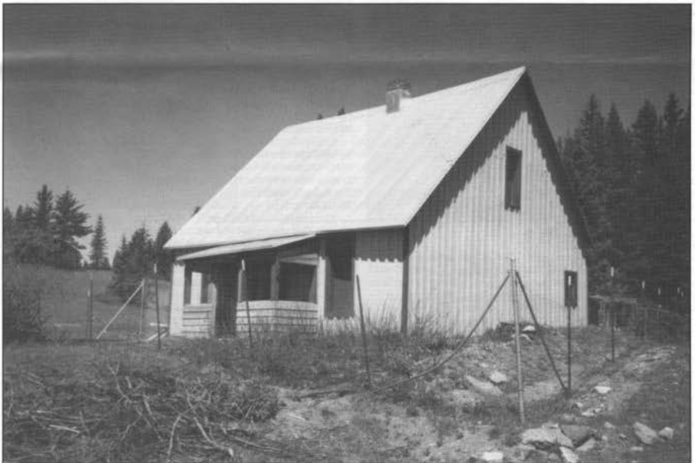
The car inspector's house is shown here in 1992 at the end of the first summer work session. The wooden footing for the front (north) porch had been rebuilt and the porch, with new siding, had been reattached to the house. The final work on the building in 1992 was installing a galvanized metal roof, the cost of which was shared with the Railroad Commission. The building had now been saved.
