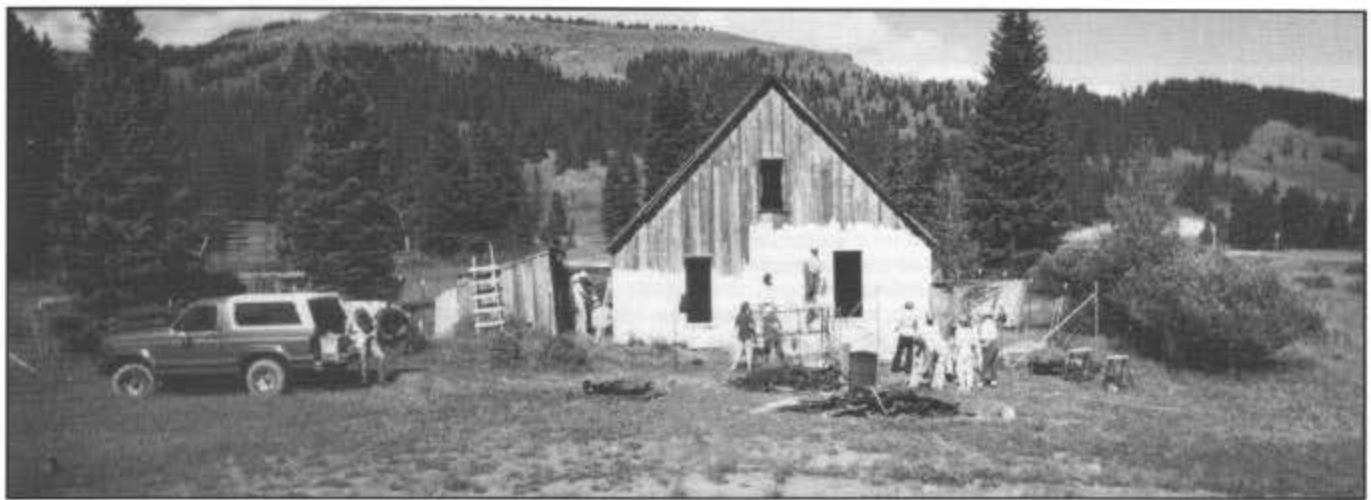
More work was done on the house during the 1991 work sessions. Volunteers completed the south-facing temporary roof and did much work on the exterior siding and battens. They also did many interior structural repairs. The crew is shown here priming the west wall; later they painted the house saffron yellow with brown trim. The snowshed can be seen in the left background.
