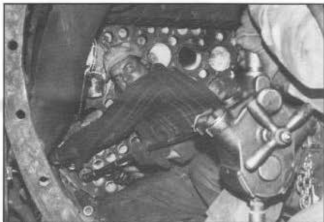
Inside the 463's smoke box, Donald Martinez guides the air-driven wrench that rotates the roller, expanding a boiler tube within its tube sheet. Open sheets can be seen just above the wrench.
