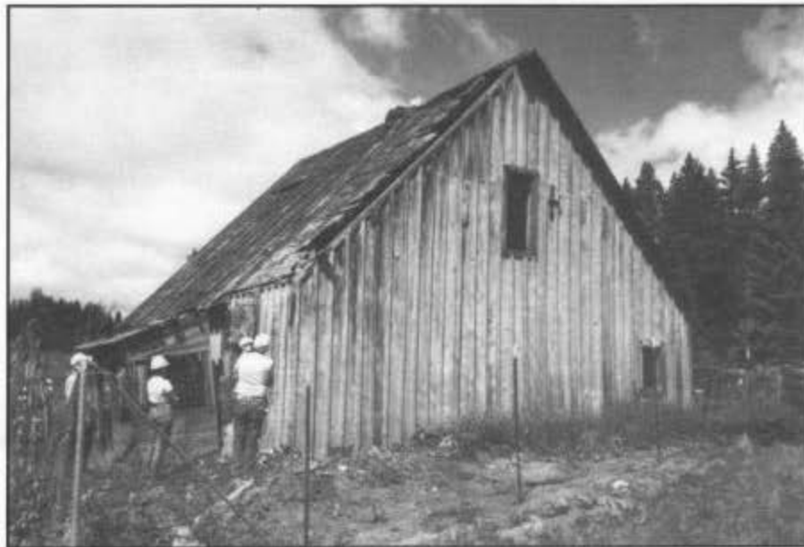
Volunteers survey the south-facing roof and the east wall in 1990. The fence was erected to keep curious persons away from the unstable structure.
