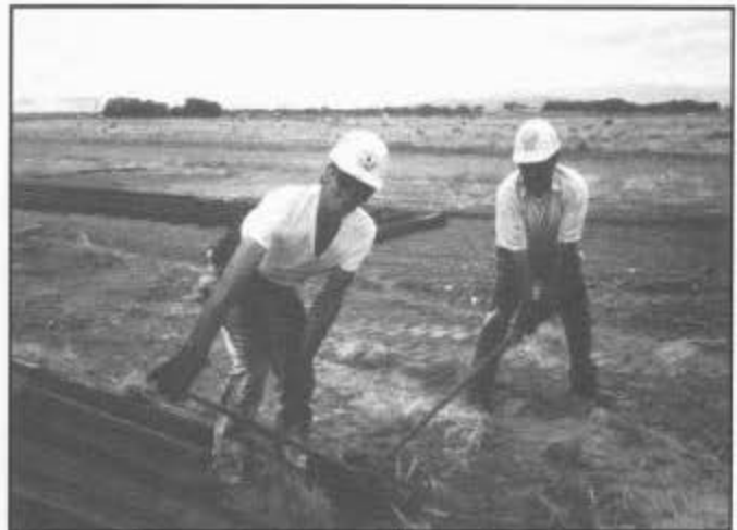
Kyle's track foreman Max Pacheco (right) assists Friends volunteer to lift a rail in preparation for setting it in place on new ties for the Antonito RIP track, July 20, 1994.
