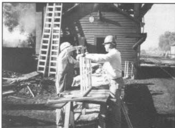
The Smucker family took on the project of the coal tipple house for the second year. Here father and son are working on replicating the original windows, July 22, 1994.
