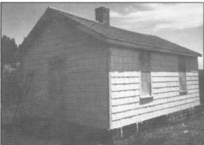
Painting in the historic abandonment white and abandonment green was almost completed at the end of the first work session. These colors were chosen to represent the last thirty years of the railroad under the D&RGW, July 22, 1994.
