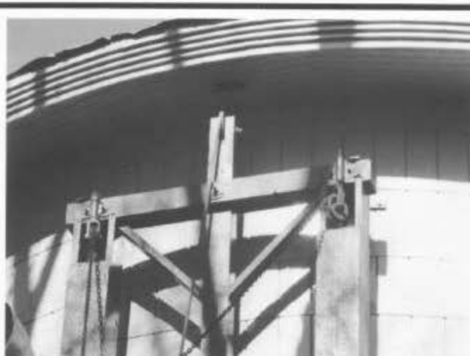
Gallows-type framework for raising and lowering the water spout and opening and closing the interior valve. June 1995.
