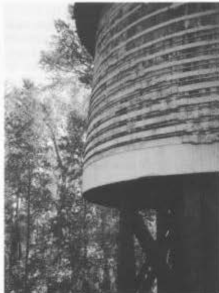
Flat bands with bolted buckles and round bars on the water tank barrel before restoration. September 1993.
