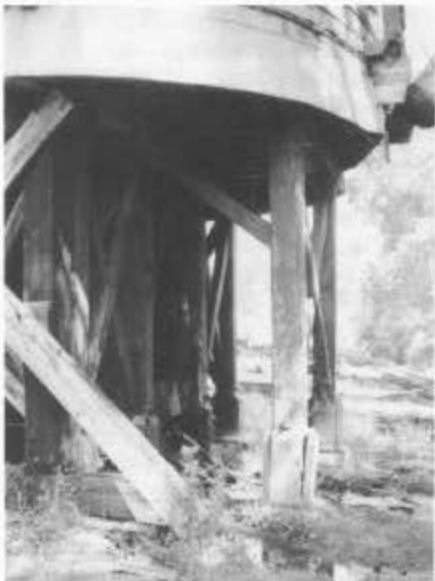
Columns with 3- by 12-inch boards at their bases. September 1993.
