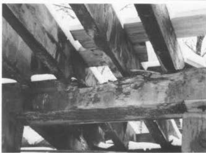
Main beams and chine joists (the wood members holding up the tank floor) showing severe rotting. October 15, 1994.
