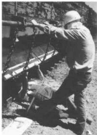
Repairing doors on a drop-bottom gondola during the 1995 summer work session. August 1, 1995, Antonito, Colorado. Photo by George Swain.
