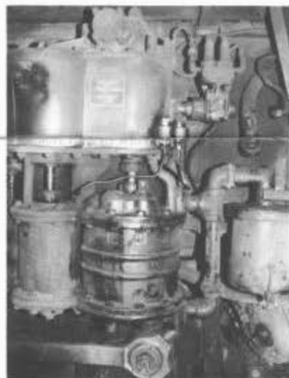
The air pump on 487. The air compressor governor is to the upper right, with the steam pipe disconnected. February 11, 1997
