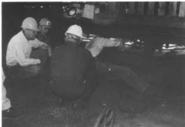
Team Leader Art Randall (left) and his second session crew talk about the brake rigging on one of the sheep cars in the Chama yard. Although the crew made significant progress on the sheep cars in the work sessions, there is no car ready to go. This is largely because the lubrication pads for the journals were not available, additional problems were discovered during the work, and the standards of serviceability have changed. The crew restored the braking systems on sheep cars 5600, 5633, and 5841. This work included changing the triple valves, repacking cylinders, renewing brake shoes, changing air hoses, and completing the brake rigging. The brake reservoir was replaced on car 5841 necessitating replacement of a part of the car floor. Train line repairs were made on the other two cars, plus other miscellaneous repairs. The sheep cars' safety appliances will require work—the cars have loose ladders and grabs. Inspection and some work was done on the other three sheep cars (5549, 5553, and 5674). On request of Chief Mechanical Officer Jack Campbell, the brake system of 5841 was measured and analyzed for braking action, comparing the results to similar measurements and analysis of the boxcar coaches, which are regarded as having good braking response. The sheep cars compare favorably.
