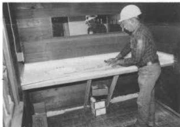
Bob Tully fits molding to the sink counter in the night watchman's house in the Chama yard. The house is being cleaned, repaired, and prepared for a summer work session bunking facility. The volunteers will restore the plumbing and install a new shower and a new gas water heater, both purchased by the Friends.
