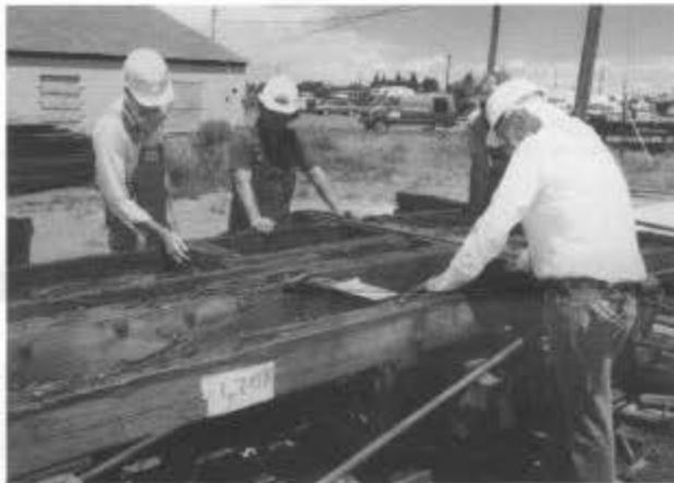
Warren Ringer (left), Bill Kepner, and Wayne Freeark look over rotten wood on flat car 6708 in the Antonito yard, August 1997. Tom Cardin photo.
