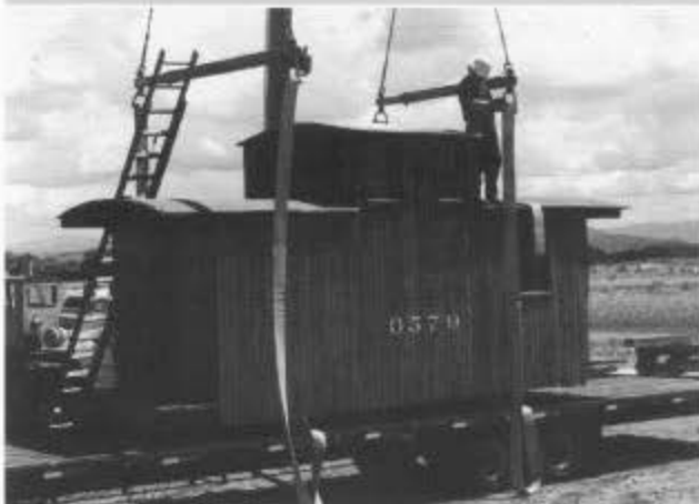
Caboose 0579 rests on a flat-bed trailer before being moved onto cribbing on the RIP track in Antonito. Once on the track, the crew began an assessment of the underframe so that restoration work can begin in 1998. To speed restoration we are looking for a second crew to plan and carry out the restoration of the roof and cupola.
