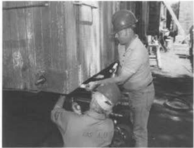
In Chama, Jay Samuels and Randy Worwag attach a plumb string to refrigerator car 55 in preparation for tightening the truss rods. The crew worked long and hard through Saturday morning to finish.
