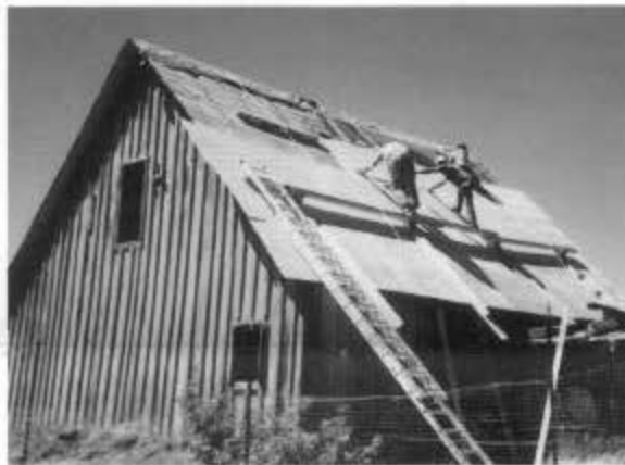
A major project of the Friends has been the restoration of the Car Inspector's House at Cumbres. Here, volunteers are replacing the roof in June 1991. Art Nichols photo.
