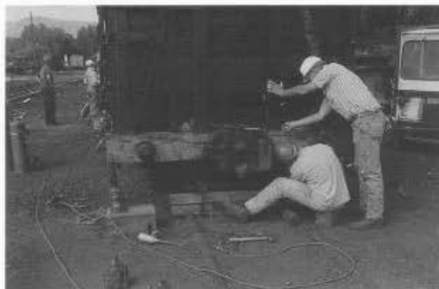
During the August mini work session, Kevin Gilbert (left) and Geof Gordon tighten bolts on the new end sill for stock car 5633. →
