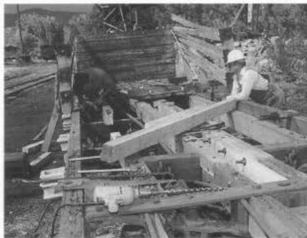
Roy Blizzard (left) and Ken Earle install new intermediate sill pieces on wheel and tie car 06092 during August 1998 mini work session.
