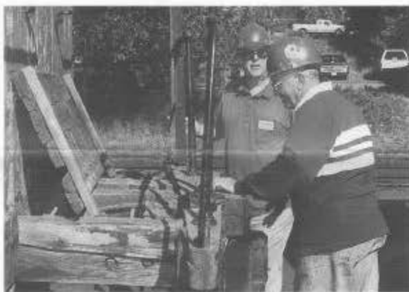
Donald Storm and Dave Sands survey the condition of the wood in the end platform of cook car 053, Chama, June 1997. Tom Cardin photo.
