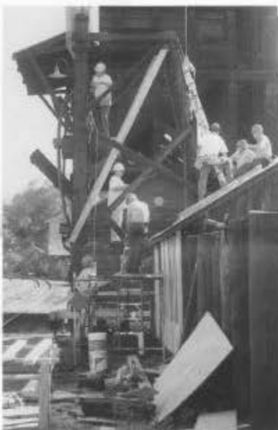
Many hands at work on the sandhouse tower in the Chama yard during the second volunteer work session, June 1997. (Tom Cardin)
