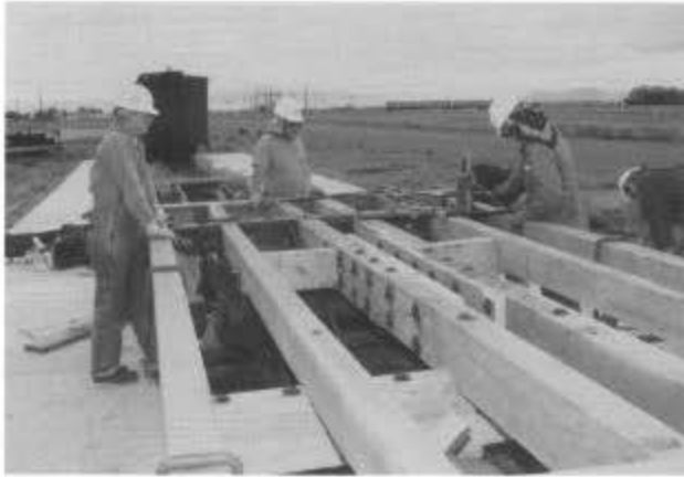
In Antonito during session A, Keith Hayes (left) and Tim Smith watch Bob Hayes use a jack to raise a timber into place so it can be bolted to the frame of flat car 6708. In the foreground, a similar timber has been bolted in place. (All photos by Tom Cardin except where noted.)
