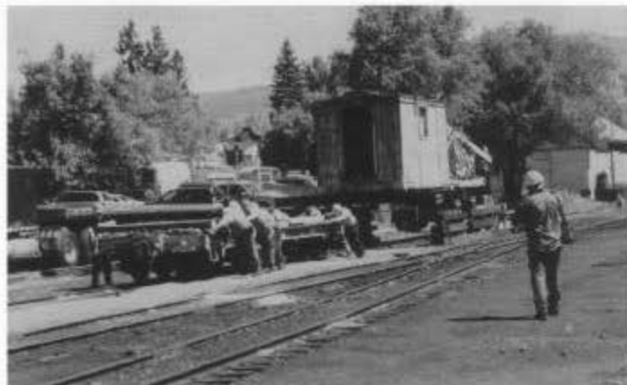
After OB's superstructure (pile driver frame, tower, hoist machinery and hoist house) was raised with jacks and supported by cribbing, the flat car was rolled out from under the superstructure (session B).
