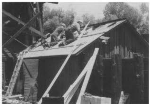
Reroofing the sand house, next to the coal tipple. Fire damaged part of the earlier roof, which the Friends installed in 1997.
