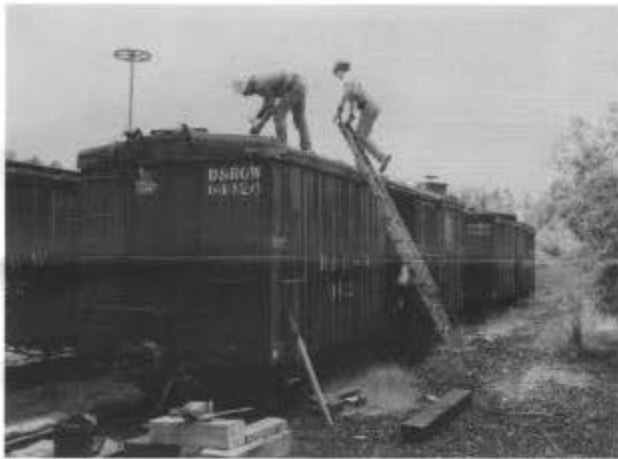
Scott Leidenberger (left) and Lisa Leidenberger work on replacing the roof walk of cable car 04426 in the east Chama yard (session B).
