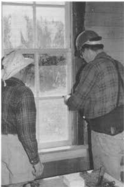
Al Judd (left) and Jerry Gorzoch hang a new window in the Cumbres section house during session C.
