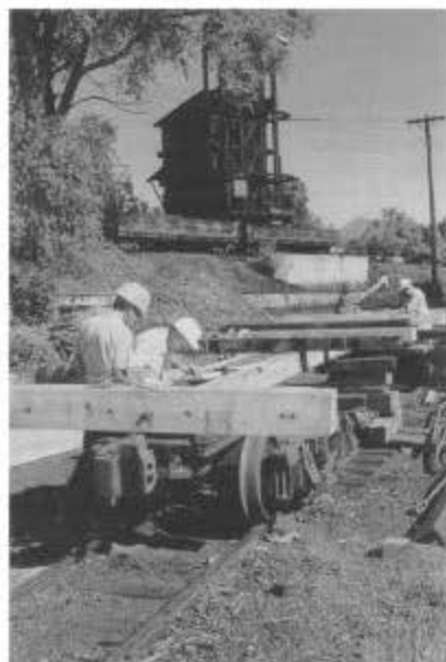
Don Bush (left) and Geof Gordon work on the center sills of flat car 6214 in the east Chama yard. In the background are Jim Phelps (left) and Fred Springer (session C).
