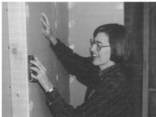
Becky Robbins sands drywall in the section house at Osier during session C.
