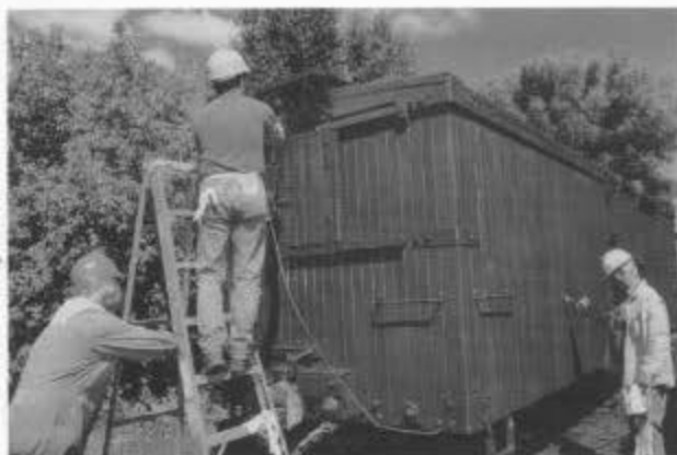
In Chama, Terry Boardman steadies the ladder while Mike Mahoney spray paints cable car 04426. In the background, John Blake brushes paint deep into the wood (session D).
