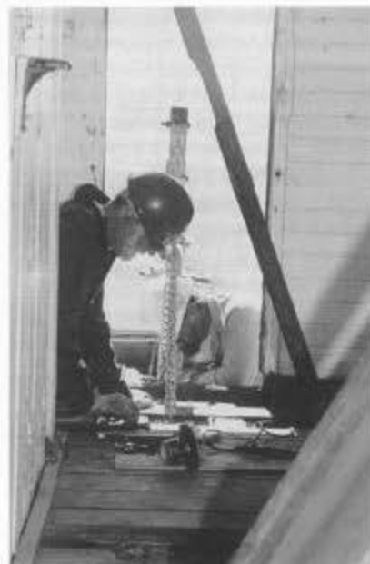
Warren Ringer (left) and Tom Garland work on short caboose 0579 during session D. They use a hydraulic lift to bring the bolster up and hold it while it is bolted in place.
