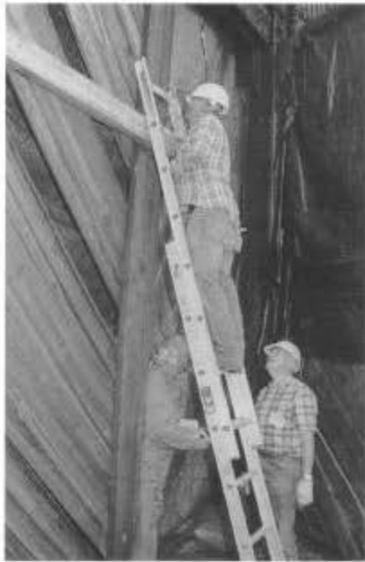
Bob Tully positions a plank on the Chama roundhouse door so it can be lifted off for repair. Terry Boardman (left) and Roger Briggs survey the situation (session D).
