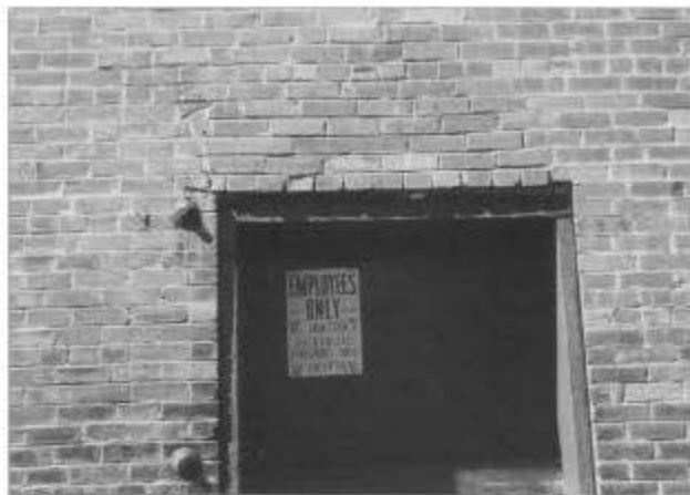
South doorway of Chama boiler room and machine shop. The single brick of the original arched doorway is above and to the left of the door. (Photos by Tom Cardin)
