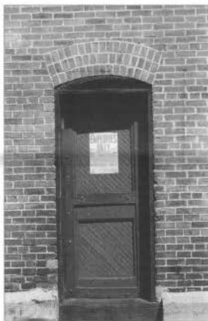
Arched doorway on the west wall of the boiler room and machine shop.
