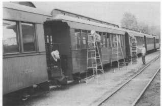
Putting final touches on coaches in preparation for opening day. Three coaches in Chama were painted. On the exterior of all the Chama coaches, loose panels were repaired and all the trim was tightened.
