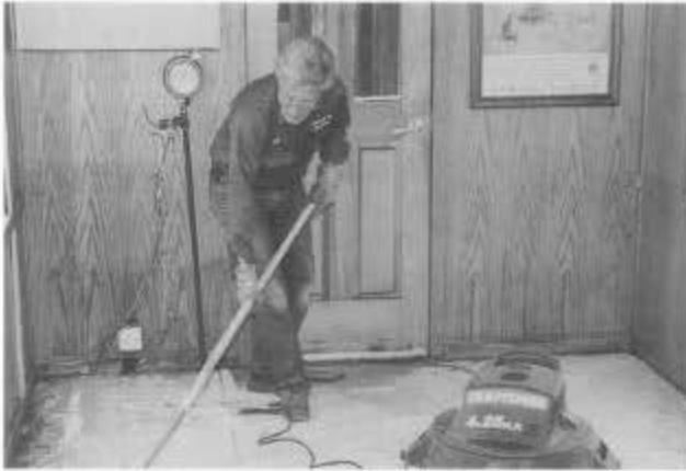
Bob Ground removes the old linoleum from Chama coach Cumbres. Volunteers then installed a new floor. They also replaced broken windows and repaired seat mounts.
