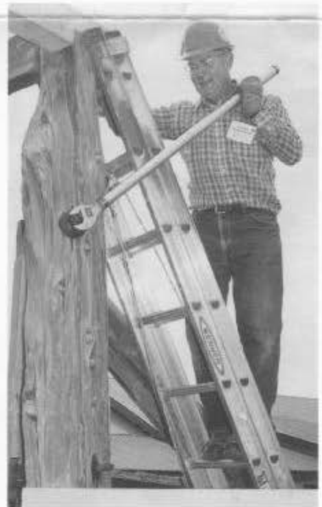
George Berkstresser uses a "cheater bar" to loosen the nut holding the hinge for one of the gates on the stock pens at the Chama wye (session A).
