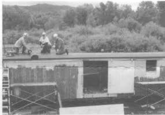
In the east yard, Bob Tully (left), Don Storm, and Donald Bayer install new roofing on water service car 04904 during session B.
