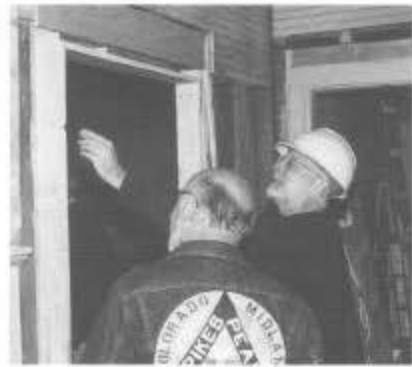
At Cumbres, Clifford Mestel (left) and Steve Schroeder check the jamb of a doorway in the section house during session B.
