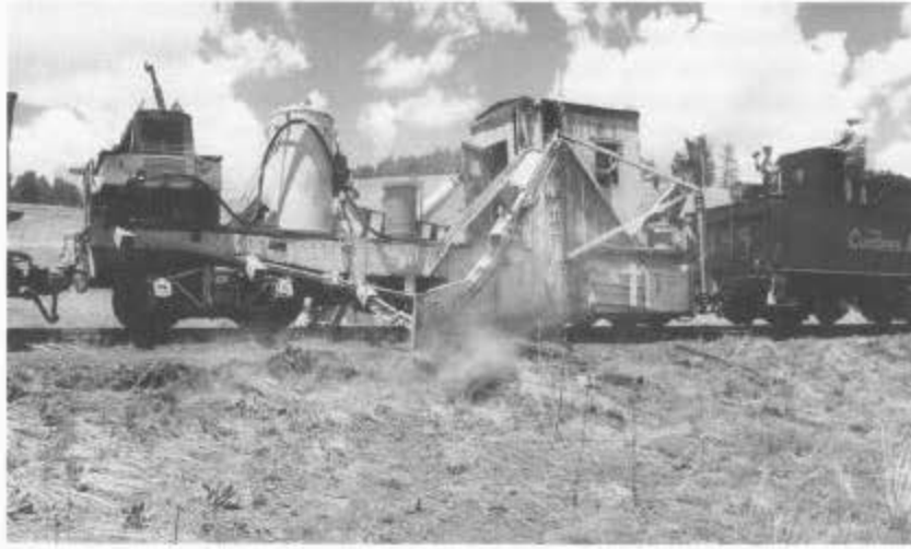
The Jordan spreader clears a wide swath along the track on June 5, 2000, as part of the railroad's extensive fire prevention measures this past year. The work extra also included engine 487 and caboose 05635. (Photo by Tom Cardin)
