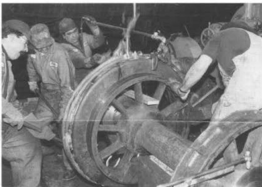
In the Chama enginehouse, the shop crew puts on a new tire for engine 463. The tire is heated with a "ring of fire" so it will expand enough to fit on the driver, with only a little coaxing from 15-lb sledge hammers. Left to right: Steve Montano, Toby Vigil, Orlando Uliberri, and Bob Wright. (March 2001.)
