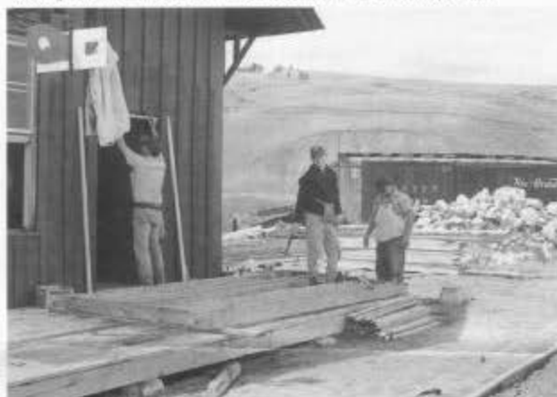
Dan Robbins (l) installs the door frame for the front door of the Osier depot while Chris Norcross (center) and Emmanuel Lopez work on the wheelchair accessible ramp (session B). The new signal mounted on the front of the depot was installed during session A. (Photo by Sheri Hamblin.)
