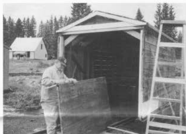
At Cumbres, John Schwartz repairs a door panel to the speeder shed. The volunteers repaired and stabilized the shed during session A. (Photo by Art Nichols.)
