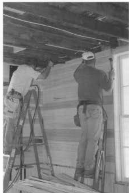
Inside the Osier depot, Dan Robbins (l) and John Ruhr fit the final bead-board strip on the wall of the first floor. The chair rail and beadboard on the ceiling are yet to be completed (session B). (Photo by Sheri Hamblin.)
