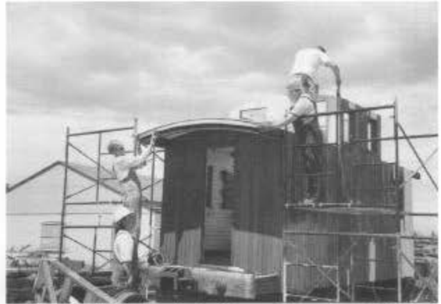
In Antonito during session A, Warren Ringer (l) and Jim Rhinehart install a curved "nailer" board on the roof end of short caboose 0579. Bill Kepner on the ground helps center the board, and Charlie Irvin works on the cupola. (Photo by Art Nichols.)
