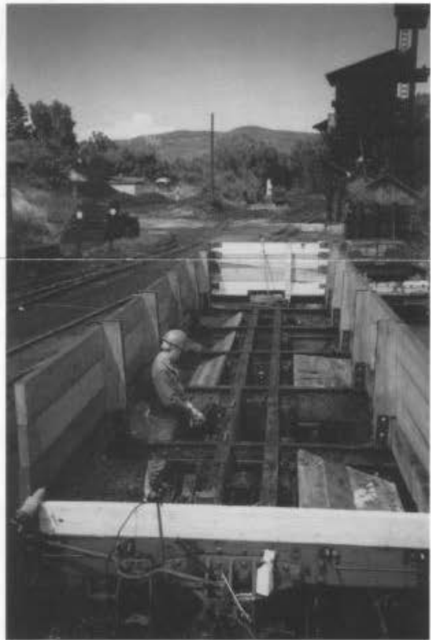
Looking north in the Chama yard, work session C, August 8, 2001. The restoration of drop bottom gondola 727 is almost complete. (Photo by George Swain.)
