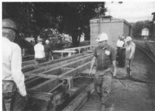
On the final day of session C at Chama, Bob Tully inspects boxcar 3339 (former coach 200) with side sills removed. (Photo by George Swain.)
