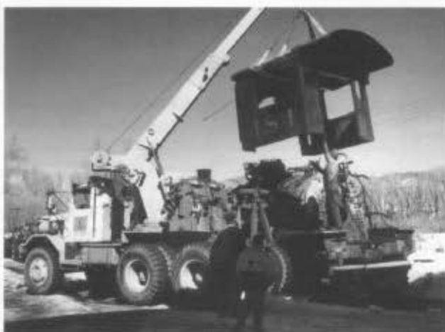
Removing the cab from 484 requires a bit of extra equipment. Steven Butler guides the cab to clear the boiler and valves. The cab must come off to get to the staybolts. Originally there were doors on both sides, but they were riveted and welded shut many years ago (February 2002).
