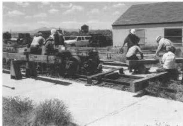
Volunteers working in the Antonito railyard. The concrete pads on both sides of the RIP track provide a clean, safe, and comfortable work area. Ft. Knox is in the background. (Photo by Tom Cardin.)
