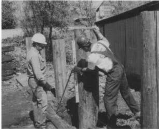
Jerry Sahnd eyeballs, while John Sutkus uses a level to set posts for the coal bunker in the Chama yard (session B). Emery Maez, general manager of Northern Rio Arriba Electric Cooperative, provided a truck and crew that drilled the holes for the posts, 16-inch-diameter, used, telephone poles that had been in the north yard. (Photo by Tom Cardin.)
