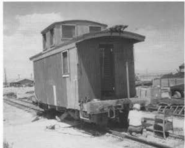
Short caboose 0579 in the Antonito yard during session C. The crew is installing the coupler on the B end of the car (the coupler pocket has been attached to a new oak end beam). Note the new wood siding.
