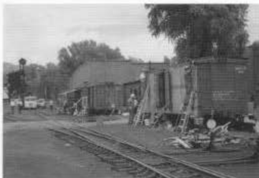
Crew members work on short refrigerator car 55 in the Chama yard during session E. (All photos by Tom Cardin except where noted.)
