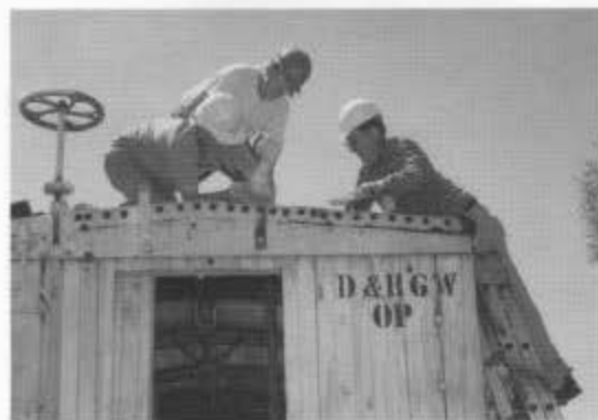
Dick Seelye (l), Grant Harrison, and Charles Joerg remove plumbing from the top of derrick OP so that they can put down weatherproof roofing material (session F).
