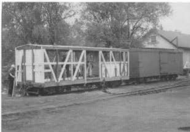
The conversion of passenger coach 200 back to its original 3339 boxcar configuration underway in the Chama yard during session C. Next to 3339 is boxcar 3605, converted from coach 209 in 2001 and ready for lettering.
