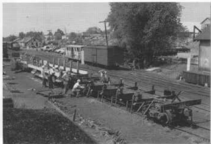
Drop bottom gondola restoration underway in Chama during session C. To the left is car 791; the crew starts to install new doors and siding. To the right is car 811 stripped to the metal frame. Boxcars 3339 and 3605 are in the center background.
