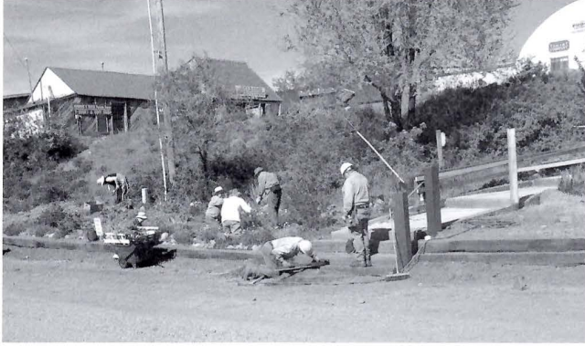
The landscaping team at work in the Chama yard and volunteers installing a handrail for the new concrete walkway from Terrace Ave. to the yard (session B).
