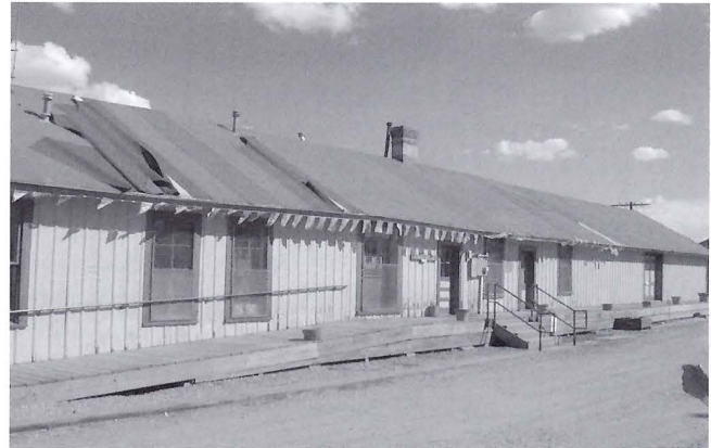
West side of Chama depot roof before repairs, showing deteriorated condition (session A).
