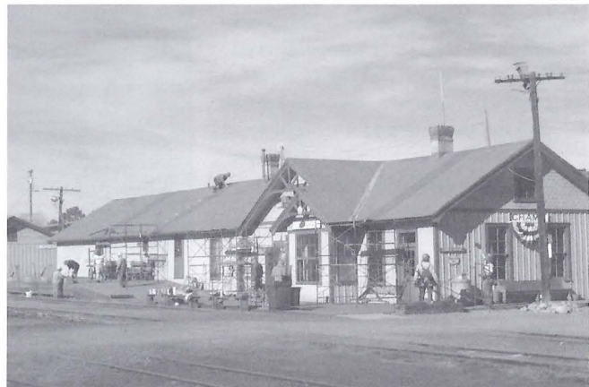
East side of Chama depot roof with volunteers making repairs (session A).
