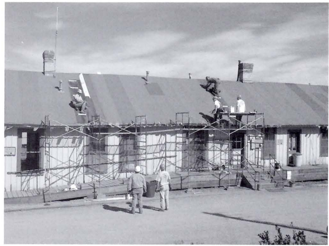
West side of Chama depot with volunteers making roof repairs (session B).
