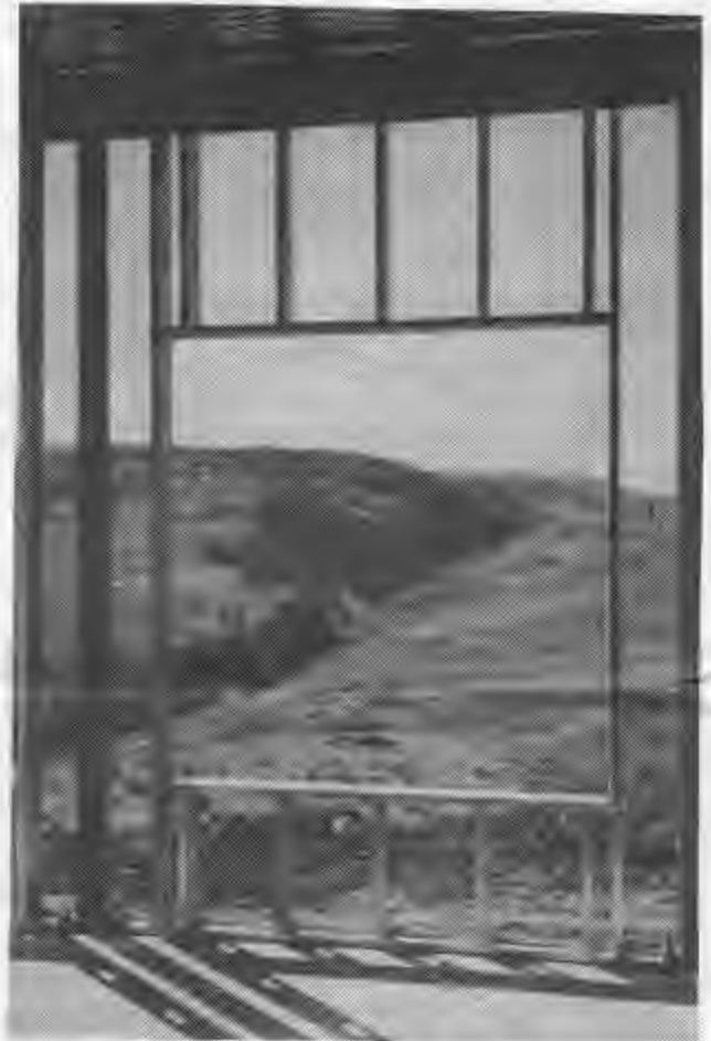
What a view to the west up the Los Pinos Valley from the lower floor of the new Dining Facility. Window framed Sept. 1988
