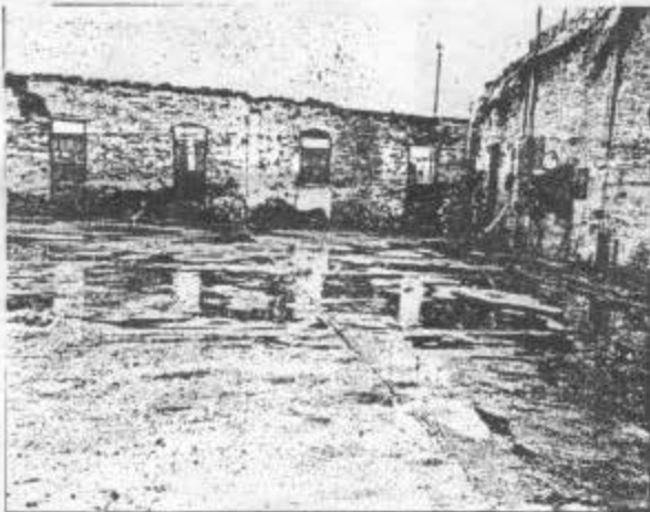
MELTED SNOW, left, reflects from the walls and floor of the gutted machine shop in the roundhouse. All the tools also were destroyed in the early-morning blaze. Machinist Les Welch, below, works in the makeshift machine shop built after the fire on the west side of the roundhouse shell. The metal lathes pictured came from Albuquerque.
